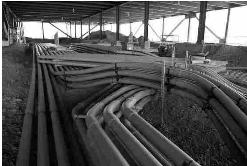
Figure 1.1: Underground Electrical Conduit in Data Center Construction
